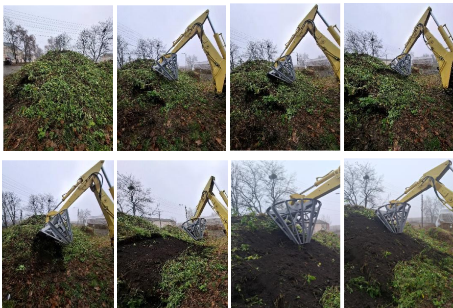
Fig. 5. Sequence of the process of removing the damaged soil layer by the working body
