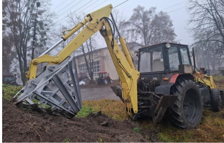
Fig. 4. General view of the excavator with the working body installed whilst removing a layer of soil
